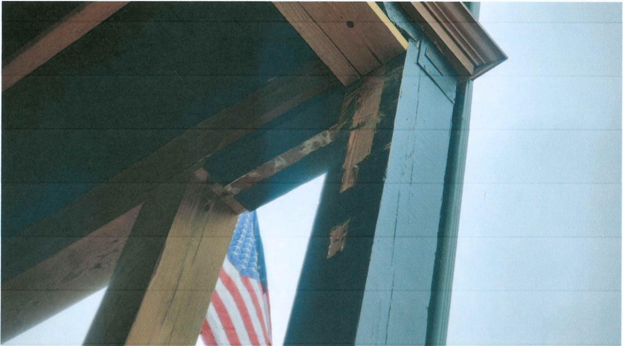
Photograph 5: Missing Historical Decorative and Structural Wood Carpentry
