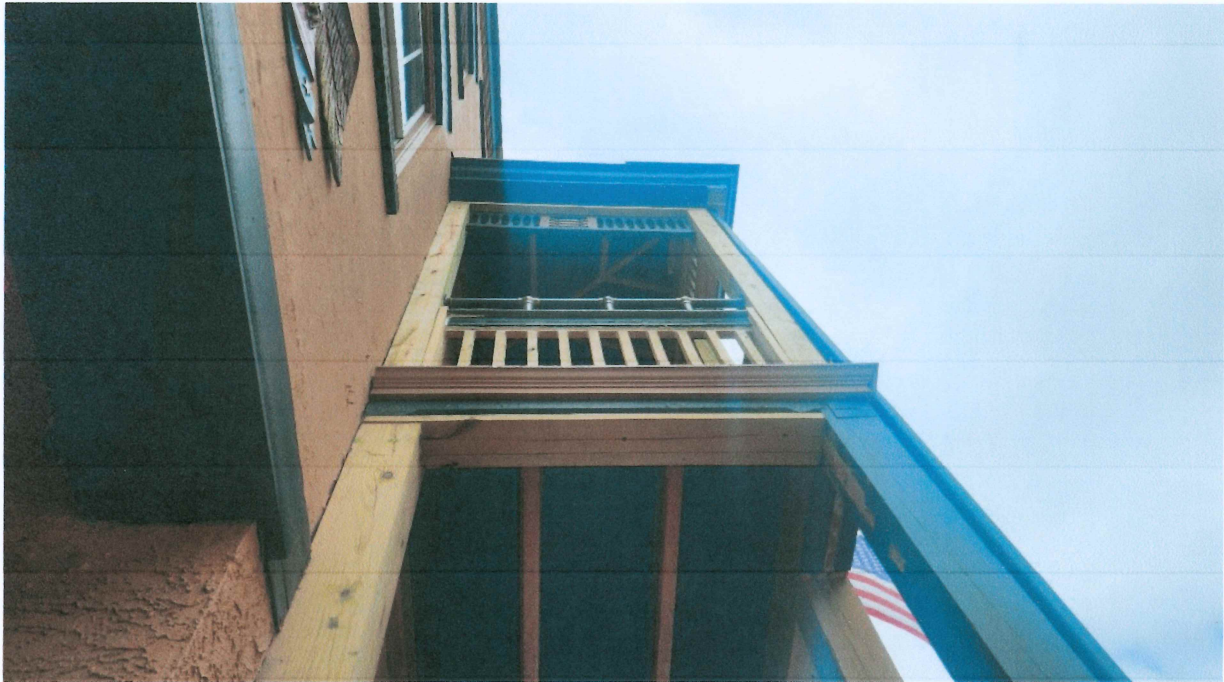
Photograph 3: Missing Post to Post Tie-down Straps
