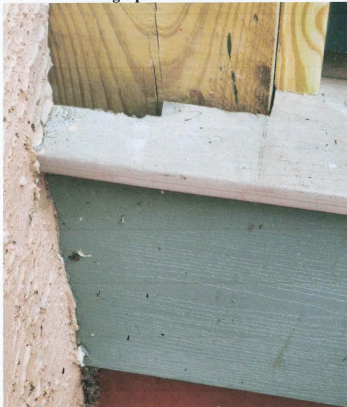
Photograph 2: Post Base Connection Missing
