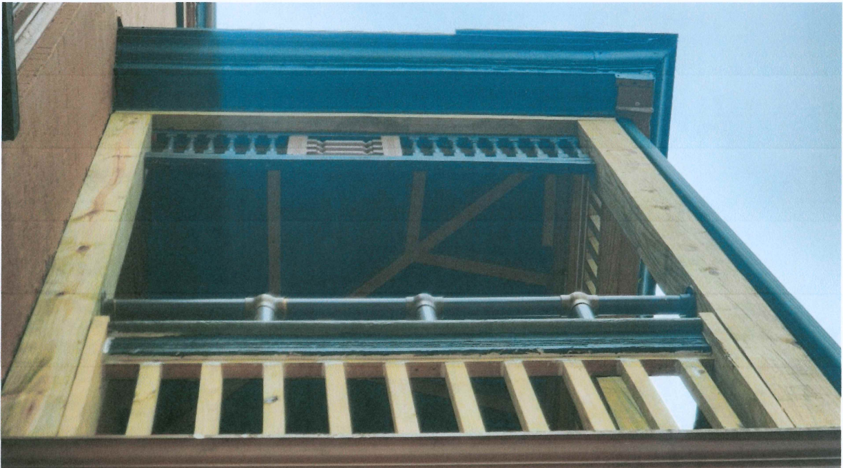
Photograph 4: Spandrel Beam and Railing Lattice Missing Gauge Clip Angles
